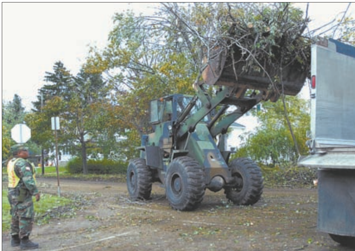
U.S. Army National Guard troops use heavy equipment to clear storm debris at Arend and Belmont, Williamsville, on Oct. 18. Sgt. Corey
